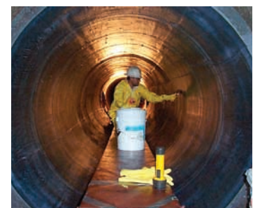
Specialty scaffolding is designed to span the spool length to allow access to the entire pipe face
